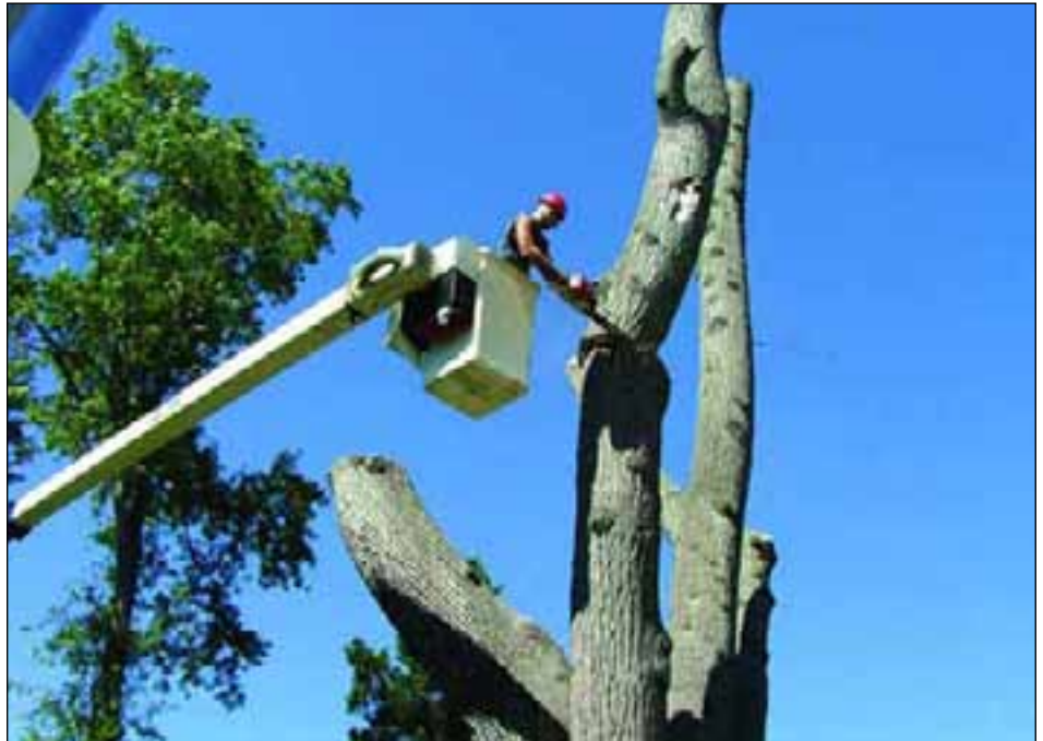
Aerial devices can provide safer, less fatiguing operations than climbing – as long as they are maintained, inspected and used according to manufacturer's specifications.
