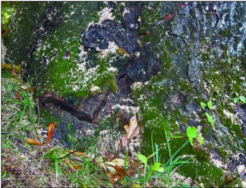
Here is a horizontal crack in a buttress root of a large hickory; the crack extends across the entire root and continues into the trunk. Notice, too, the amount of decay in the root where it is cracked. This is a very dangerous situation.
